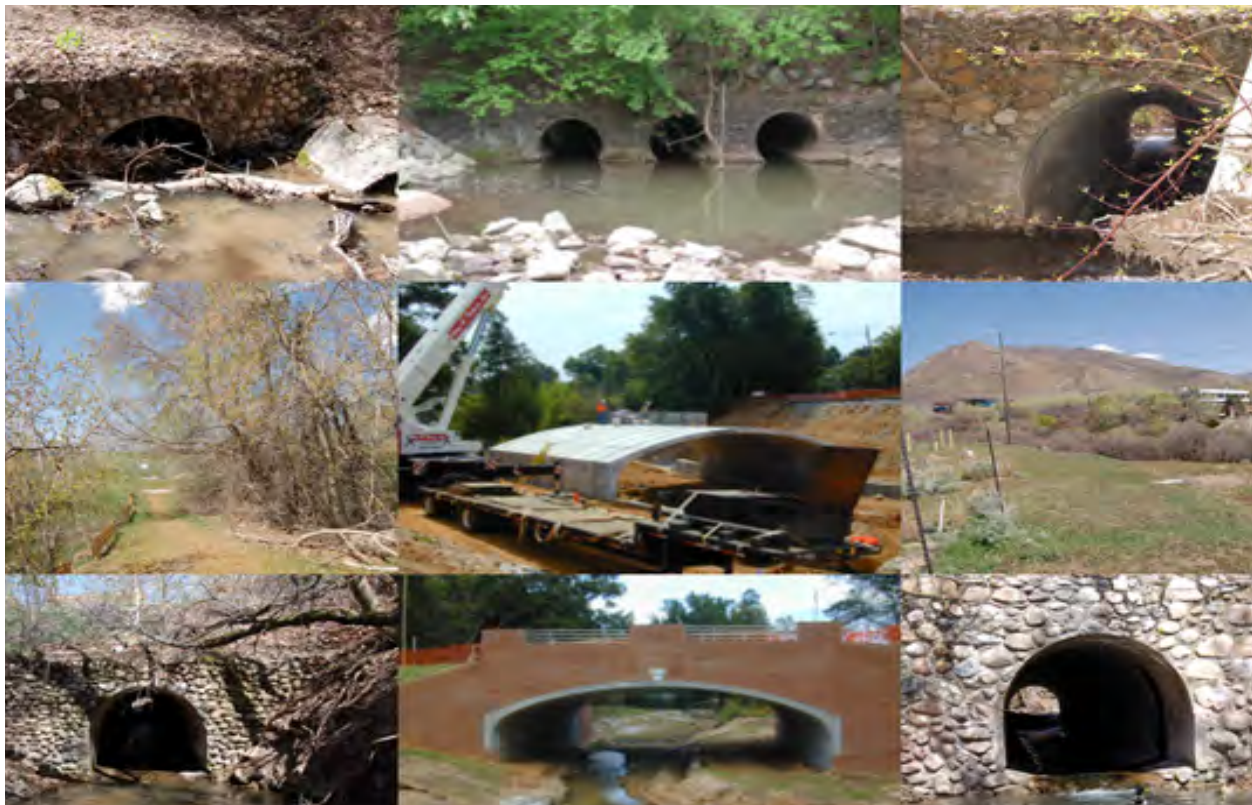
Figure 5.13: Side Panels - Closed culverts and bridges along RBC Center Panel - Replacing a closed culvert with an open arch design at North Carolina State University
